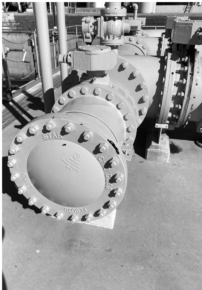
PHOTOGRAPH OF SECONDARY EFFLUENT NOT TO SCALE
