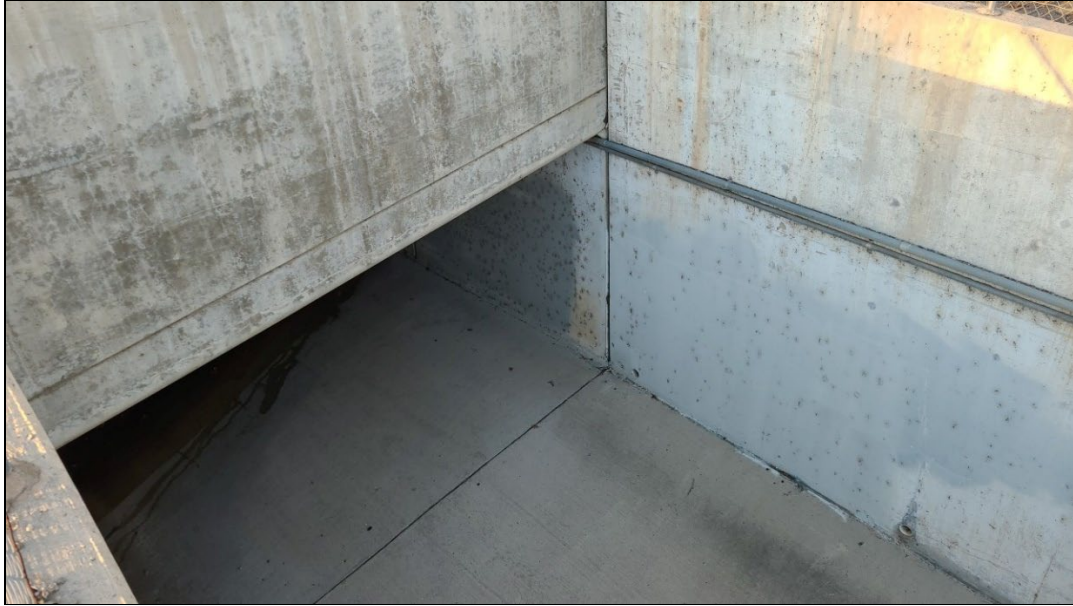
Photo 11: Concrete box culvert in concrete-lined drainage channel located within the Project Site, under West Ontario Avenue and west of Oak Avenue, facing south.
