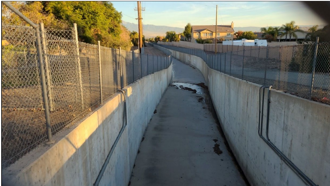
Photo 12: Concrete-lined drainage channel that intersects the Project site, under West Ontario Avenue and west of Oak Avenue, facing north.
