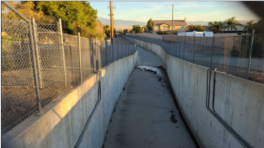
Photo 12: Concrete-lined drainage channel that intersects the Project site, under West Ontario Avenue and west of Oak Avenue, facing north.
