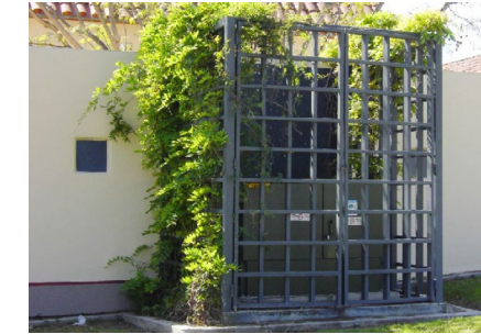
Attractive screening of mechanical equipment
