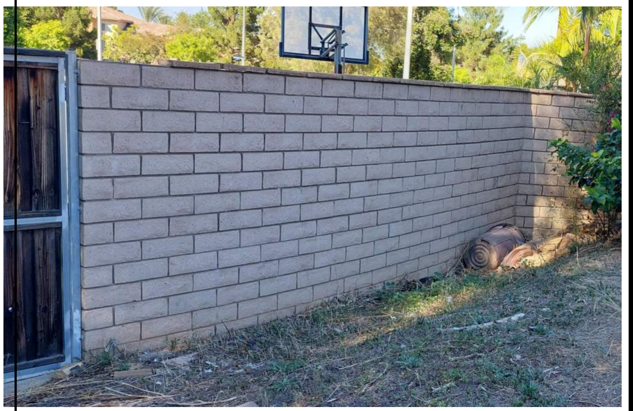
EXISTING BLOCK MASONRY WALL ON THE NORTH & WEST SIDE. BELONGS TO THE HOA -TO REMAIN.
